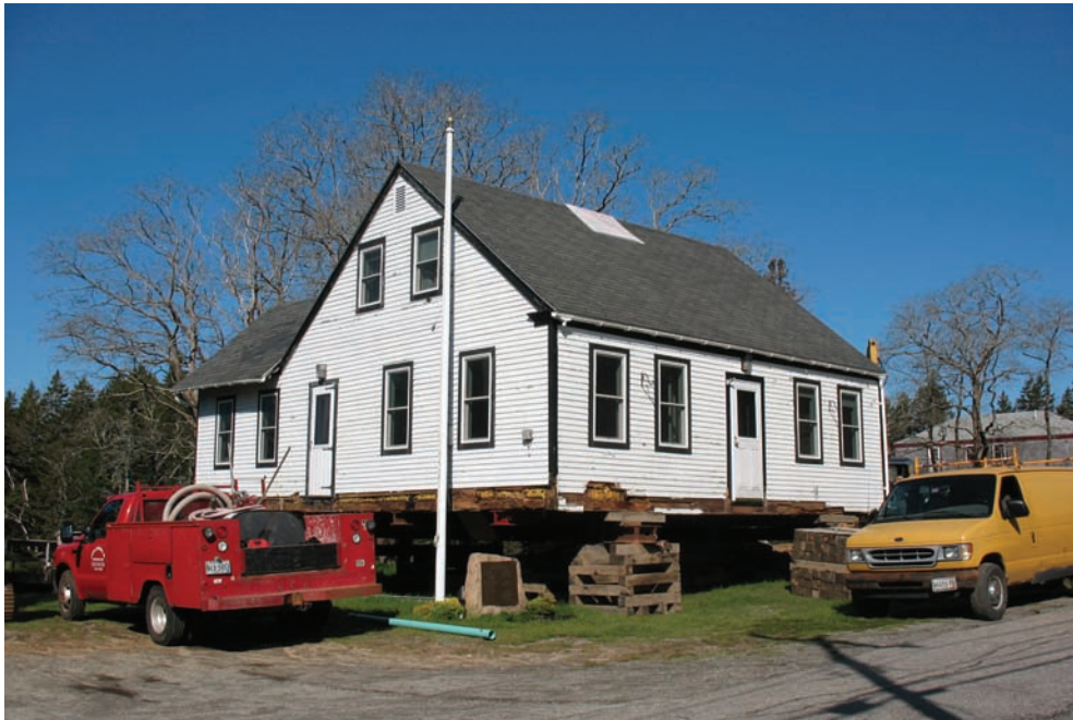
Parsonage renovation. In 2013 the parsonage was renovated from the ground up. It was moved off its foundation and temporarily shifted thirty feet closer to the Church. The cellar and additional space under the kitchen were excavated, and a new cement foundation was poured. The house was then moved onto the new foundation and expanded. The second group of shoes was found during the cellar renovation. Photograph by the author
