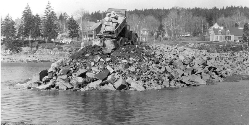
In January 1954, a stone-walled bulkhead was built across Frazier's Cove. Courtesy of the Northeast Harbor Library
